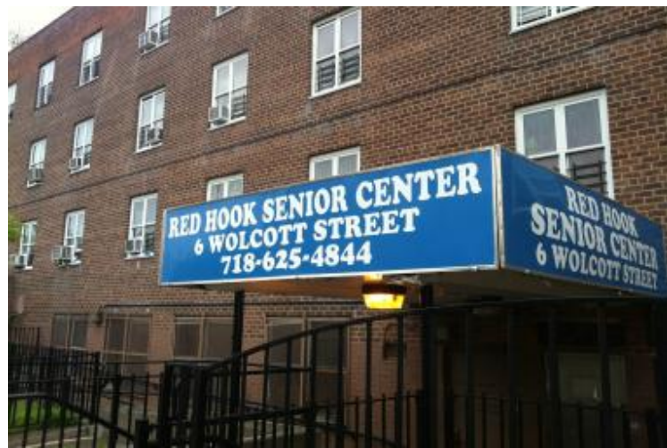
The former location of the Red Hook Senior Center at 6 Wolcott Street has been abandoned for ten years, after taking critical damage from Hurricane Sandy. During the early days of the pandemic in 2020, a tenant living above informed the author of this report that the empty space had become a breeding ground for vermin. Credit: Nikhita Venugopal/DNAinfo.
