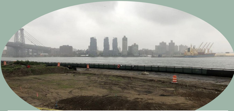
Area of where the former amphitheatre of the East River Park and was demolished for new construction
